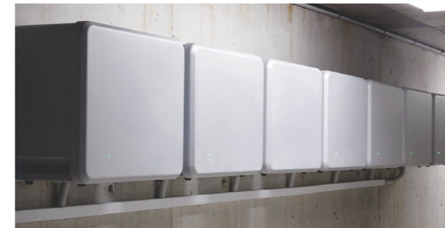
Wall-mounted lithium battery
